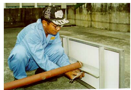
Illus. F PV module mounted on steel post and secured with a 2 inches U-Bolt
